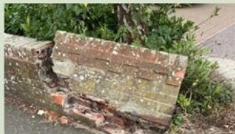
Car Park Damaged Wall 19 August 2024
